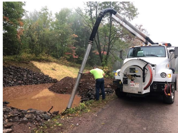
City of Hurley's vac-truck removed the water flushed through the new stream section to remove the sediment and water before connecting the stream.
