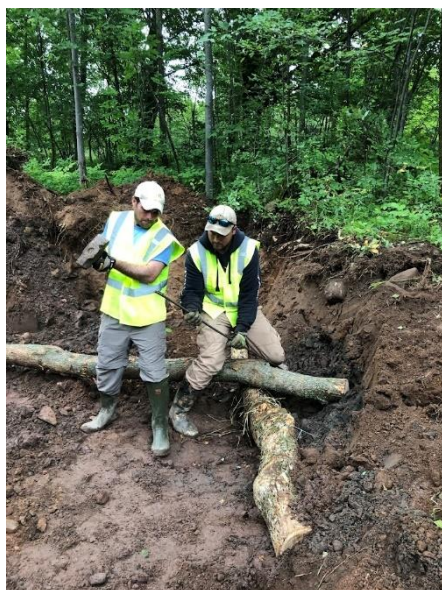
Installing a spider log for brook trout habitat in the new stream channel.
