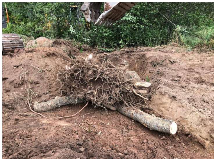
Spider logs installed on an outside bend in the new stream channel, brook trout will seek shelter under the new stream habitat.
